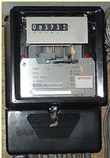
3-phase electromechanical induction meter,
